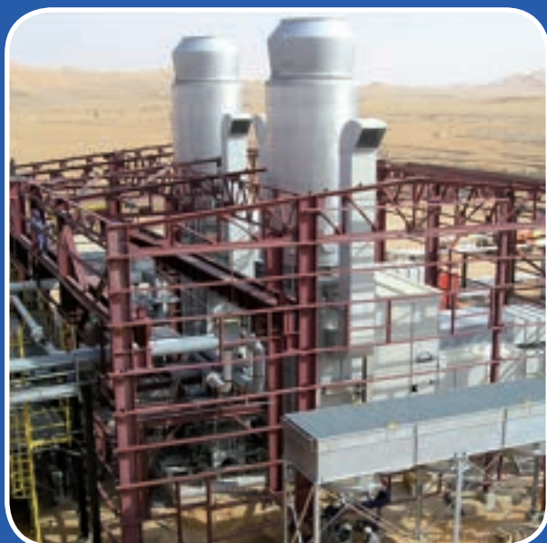
Nießing silencer systems are also used in turbines that are subjected to high temperatures
