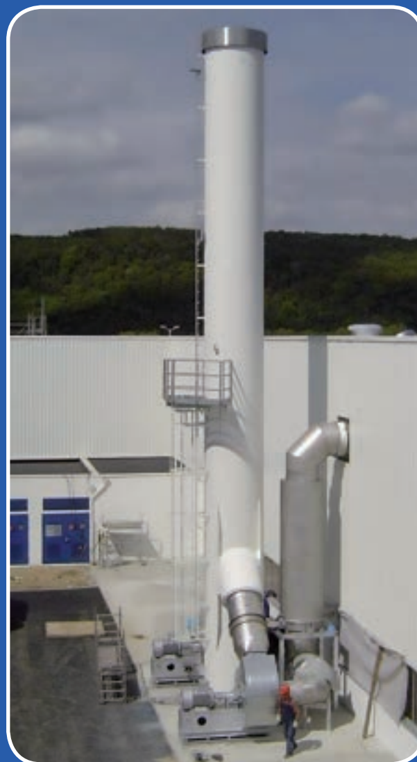
Nießing exhaust air system for Renault engine test benches
