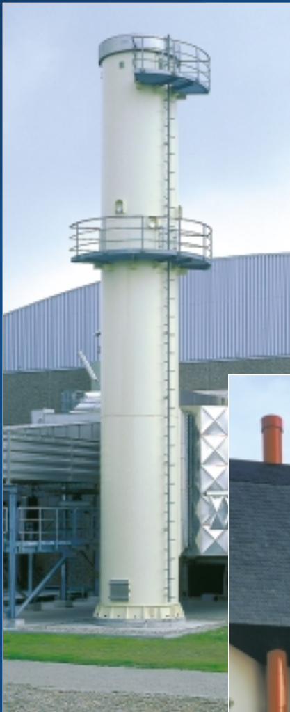
N1-SE 17 m Verdichterstation, Rysum
