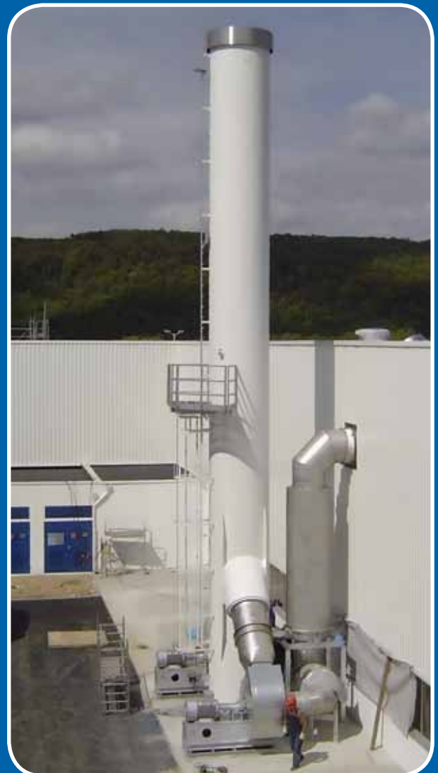
Nießing exhaust air system for Renault engine test benches
