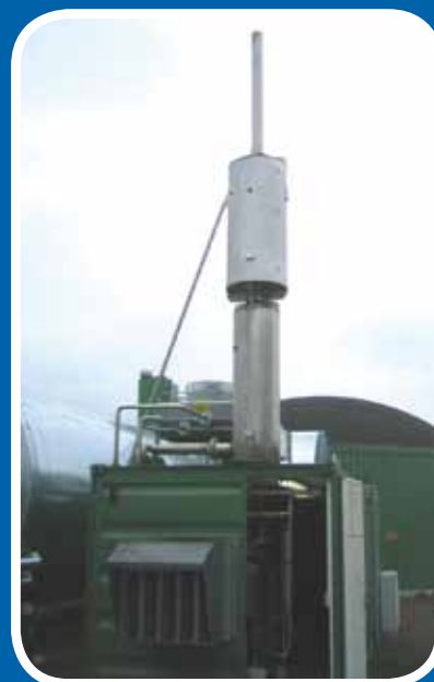
Housing for a biogas generator in a container with adequate silencer system
