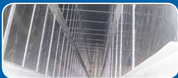
View from above into the 50 metre deep duct with installed sections of Nießing plate absorber
