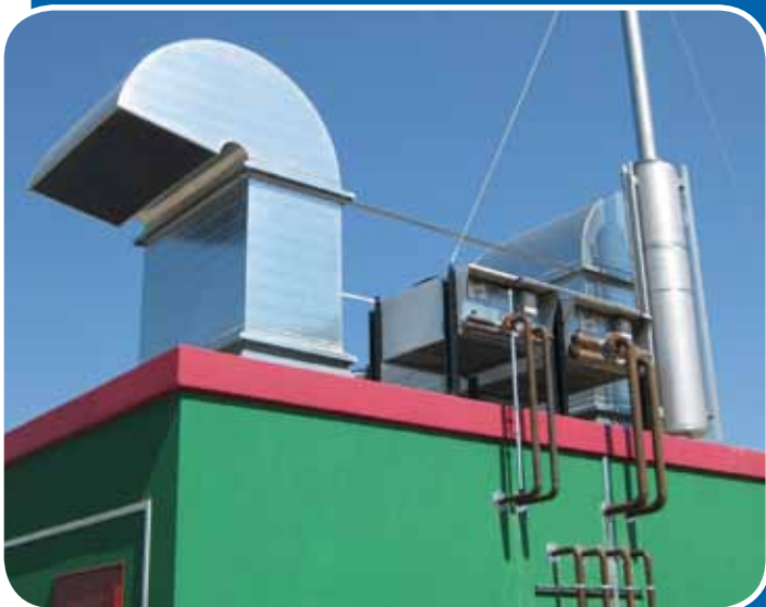
Typical exhaust gas silencer installation for a biogas plant. The main priority here is the elimination of low frequencies (engine ignition frequency)
